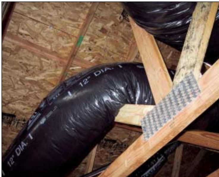
FIGURE 7. Fortunately, the HVAC installer didn't cut out the truss members to make room for the ductwork. However, this sharp bend could have been easily avoided by rerouting the duct from the start. Codes require that duct be installed fully extended, not compressed.
