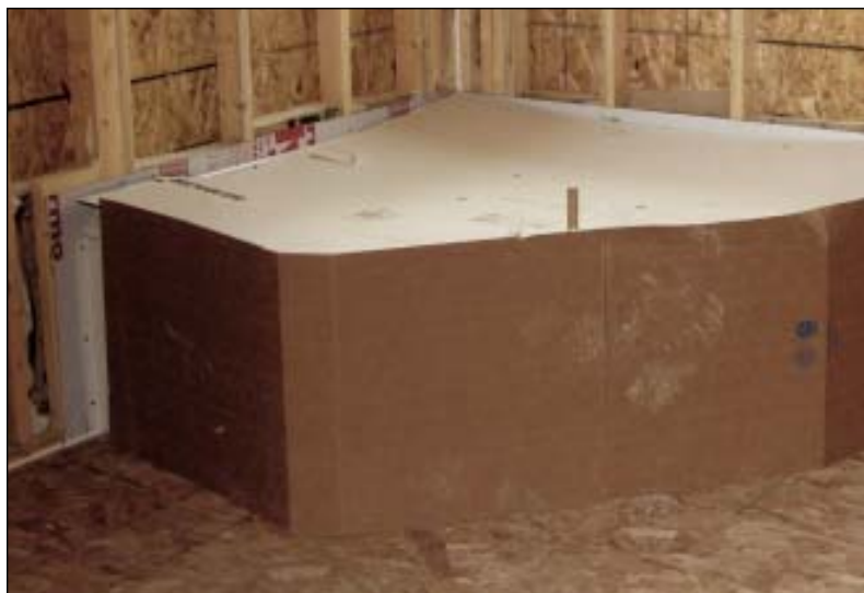
FIGURE 4. Before installing a tub unit, the wall cavity must be insulated and sheathed to stop the free transfer of air and energy. Thermo-ply or a similar type of sheathing is a good choice for this application because it doesn't pack the wall out too far.
