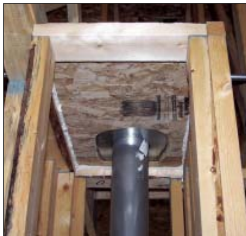
FIGURE 3. The top of a vent chase can dump a lot of conditioned air into an attic. Prior to installing the vent, cap the chase with OSB and seal the edges with a foam sealant, then seal the vent to the OSB with a metal collar.
