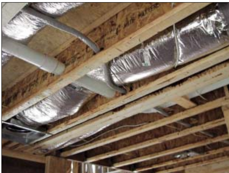
FIGURE 8. Coordinate the mechanical trades: This conflict between the HVAC duct and a plumbing drain could have been avoided by both trades meeting and reviewing the plans prior to the crews' arrival on site.
