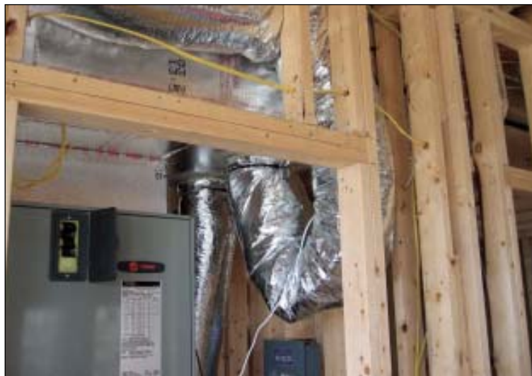
FIGURE 6. The kink in this duct will severely restrict airflow. Like a kink in a hose, the reduced size increases the pressure in the duct, causing any leaks to shoot air at a higher velocity.
