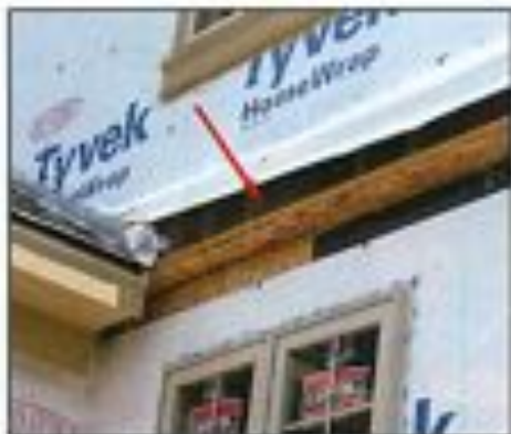
Photo 8 - Hole in water-resistive barrier (WRB).
