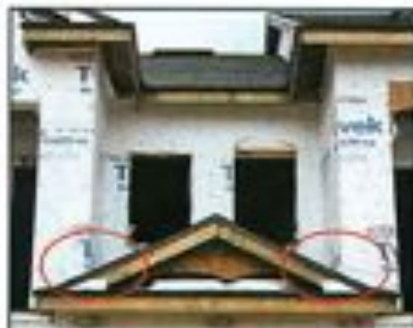
Photos 2 - Roof sloping into walls.
