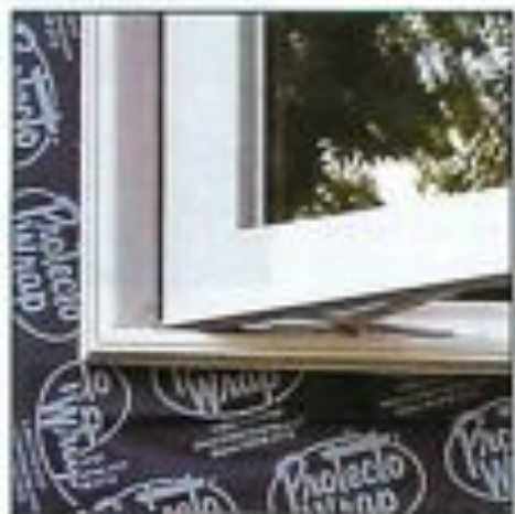
Photo 32 – Improper sill flashing.
