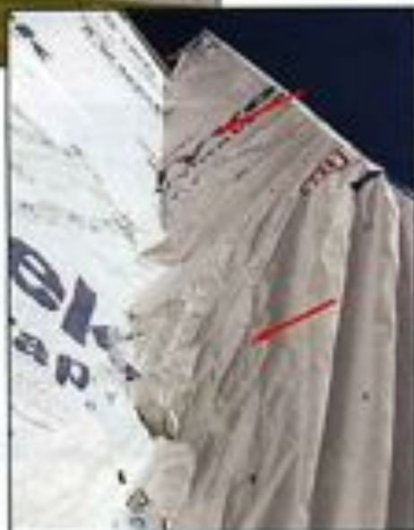
Photo 19 - Rips and gaps in WRB.
