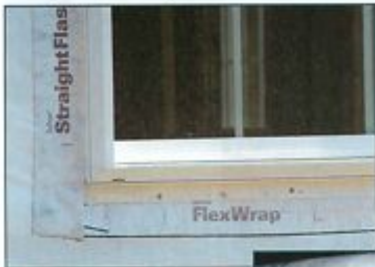
Photo 28 - Proper window flashing at sill. The sill flashing was installed before the window.
