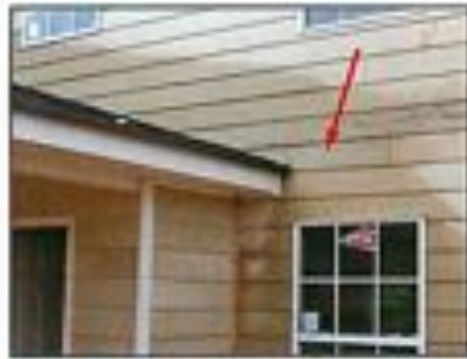
Photo 7 - Moisture at roof/wall intersection.
