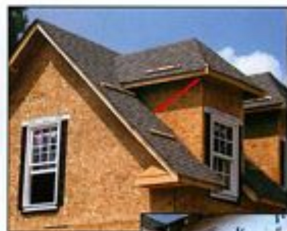
Photo 16 - Missing step flashing.
