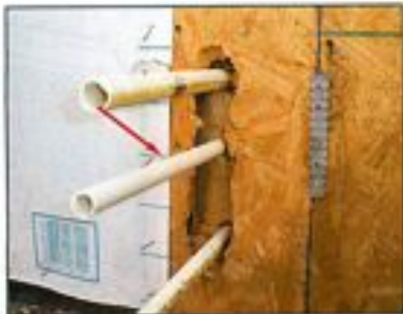
Photo 21 - No flashing around pipes.
