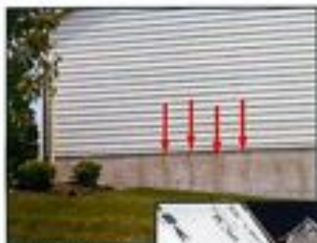
Photo 18 - Vinyl Siding Drainage
