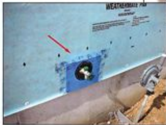
Photo 24 - Penetrations should be flashed and properly integrated with the house wrap (WRB).
