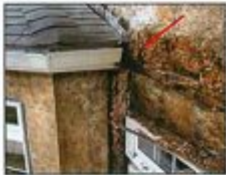
Photo 6 - Damage at roof/wall intersection.
