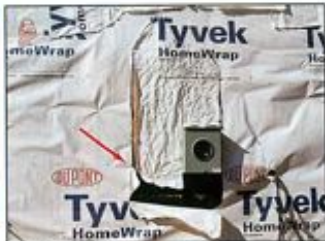
Photo 22 - Poor detailing at electrical meter.
