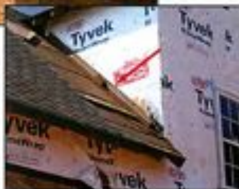
Photo 17 - Missing counter flashing.
