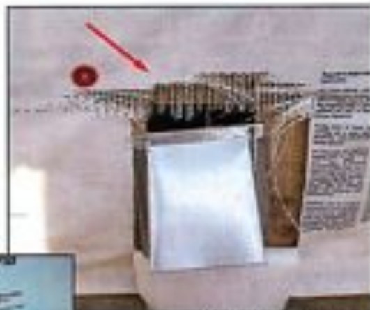
Photo 23 - WRB at vent should be flashed.
