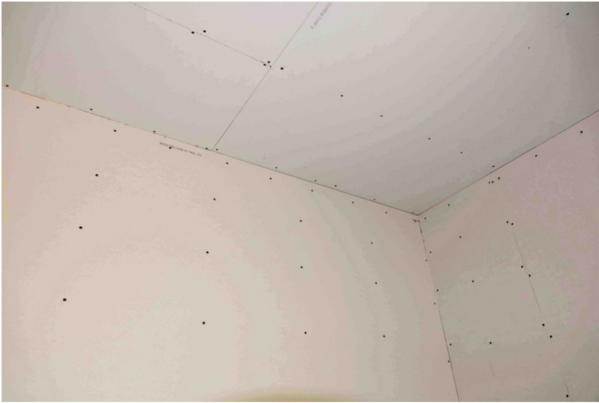
Fasteners placed tight into wall and ceiling corners may cause cracking in the corner. Instead, hold fasteners back to allow the corners to float.
