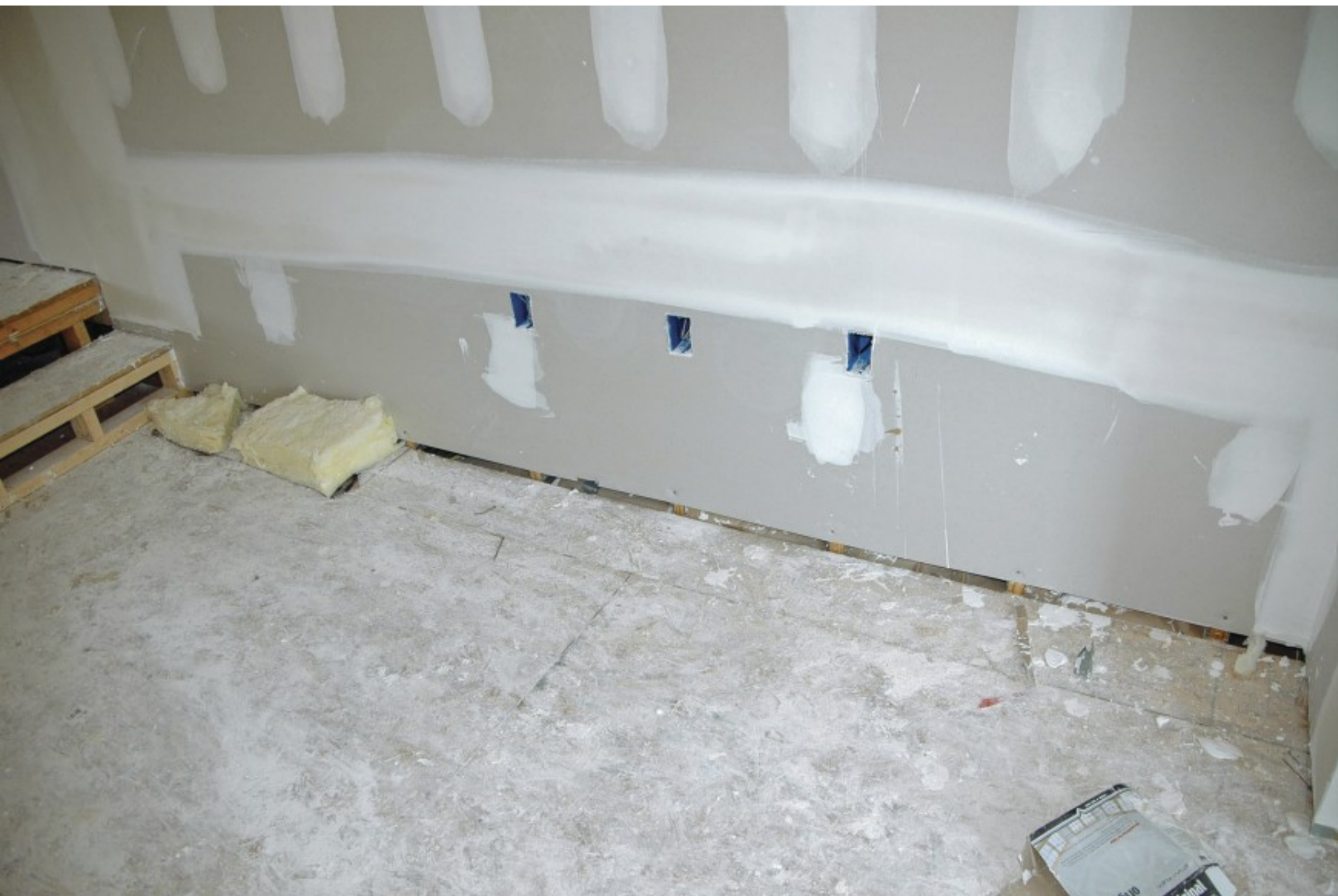
All exterior wall plates can leak, and the garage separation wall should be considered an exterior wall.
