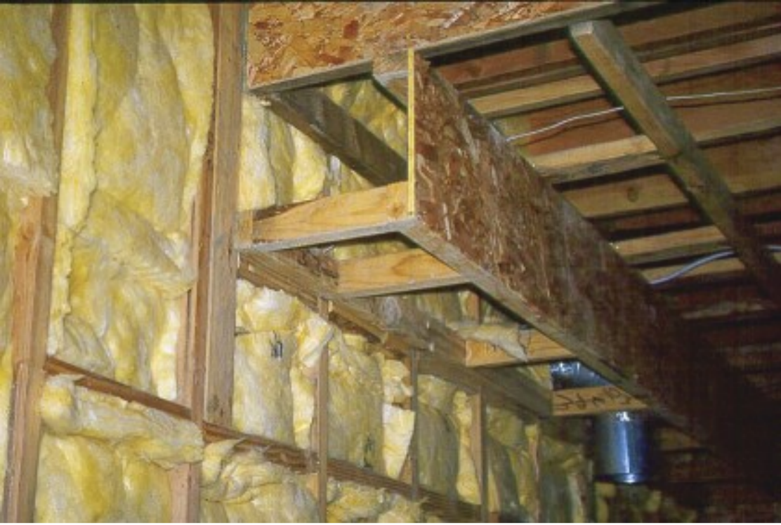
Cabinet soffits are huge leaks to the attic.
