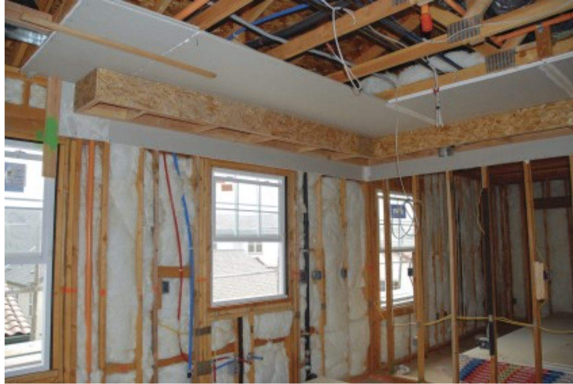
Drywall on the lid is the best way to shut these down.
