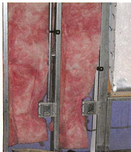
Common installation defects with batt insulation.
