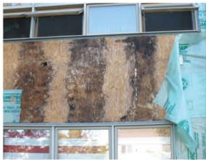
Moisture damage due to a lack of window flashing.
