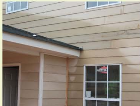
Notice the moisture loads at roof-to-wall intersections and the need for kick-out flashing.
