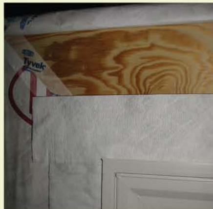
Note the head flashing correctly spans from the nail fin of the window onto the sheathing under the building wrap at the head of the window.
