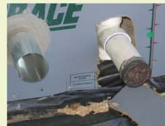
Building wraps work well keeping water out of building cavities. However, it is important that all penetrations are sealed. The penetrations shown here will surely lead to water leaks and expensive callbacks.
