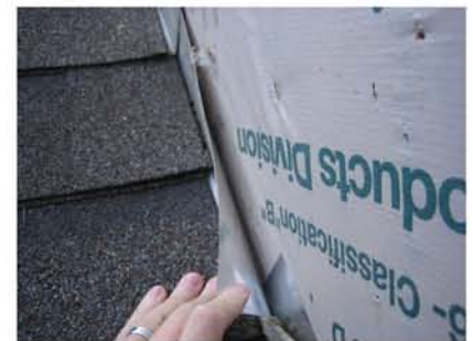
Roof-to-wall intersections are often reversed shingled as shown here. If water gets behind the cladding it will cause a leak. The wrap should go over the step flashing.
